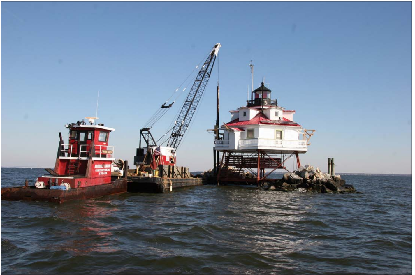
Driving the first piling for a dock at Thomas Point Shoal Lighthouse. Photo by Henry Gonzalez.
